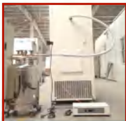
LN 2 /CO 2 backup system
